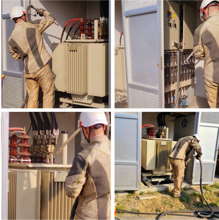
Figure 2: Dry ice blasting on power substation 10(20)/0.4 kV in Elektra Zagreb (May 2022, own photos)
