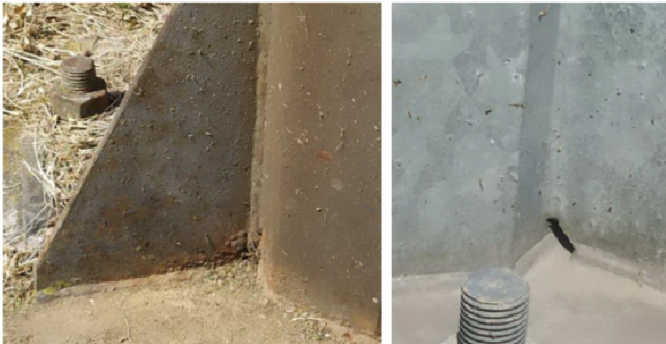
Figure 2: Base of public lighting poles in the city of Karlovac. Left - bad design; corrosion occurrence due to weld accumulation in sharp corners. Right – good design, small pockets eliminate weld accumulation and provide better drainage.
