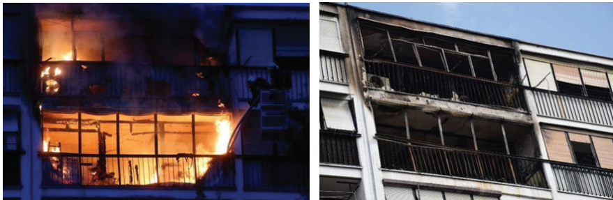
Figures 4 and 5: Transmission of fire over the loggia on the upper floor
