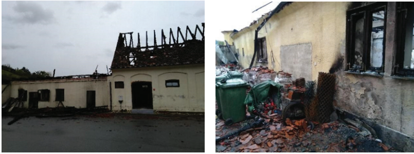
Figures 6 and 7: Auxiliary building fire and the place of the occurrence of a fire
